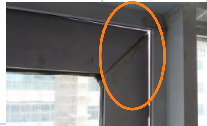
Openable window with gaps - Not sealed
