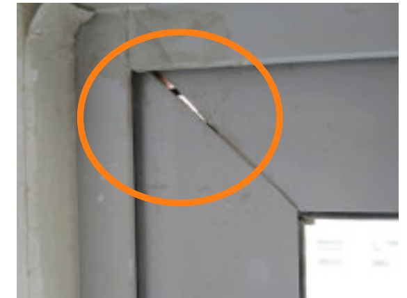
Incorrect Corner Joint- Poor Fabrication
