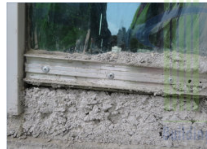
Loosely filled mortar, can't achieve good waterproofing
