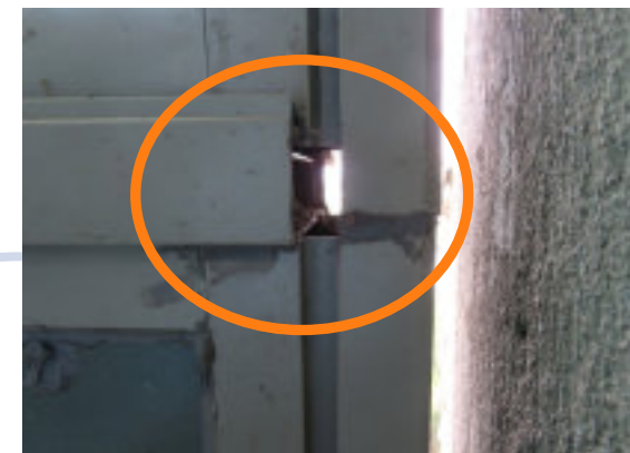
Gutter not sealed / joined at ends, holes in facade
