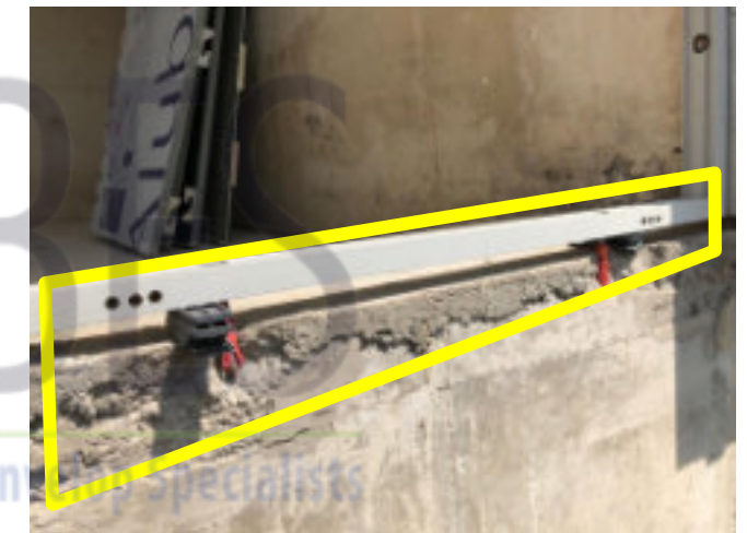
Poor Concrete Opening, Window perimeter sealing very difficult and risk of water seepages
