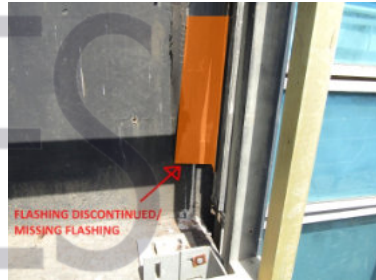
Flashing Discontinued at Interface, risk of leakages
