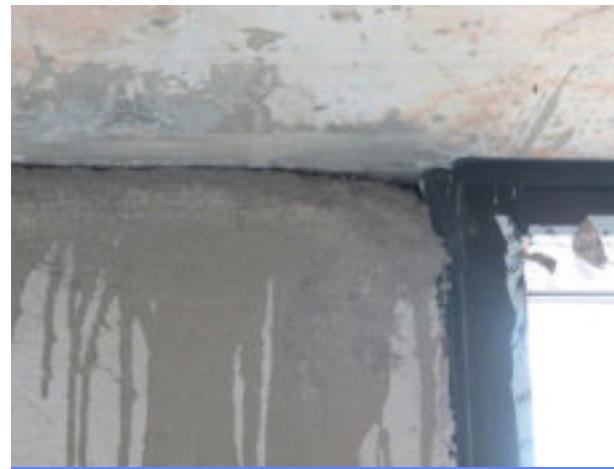
Joins not treated, leakages at wall and roof
