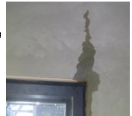
Leakage due to Cracked Concrete
