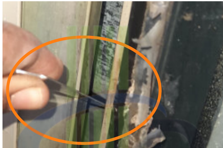
Flashing Discontinued, entry of water into joints
