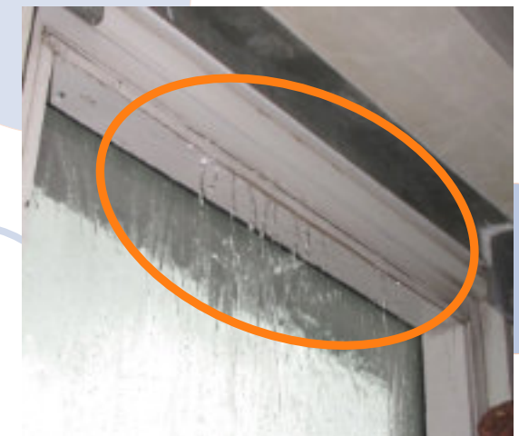
Leakage due to poor hardware & Gasket
