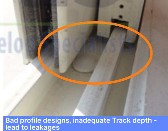
Leakage through Sliding Window in closed condition, incorrect gutter depth & Weep holes
