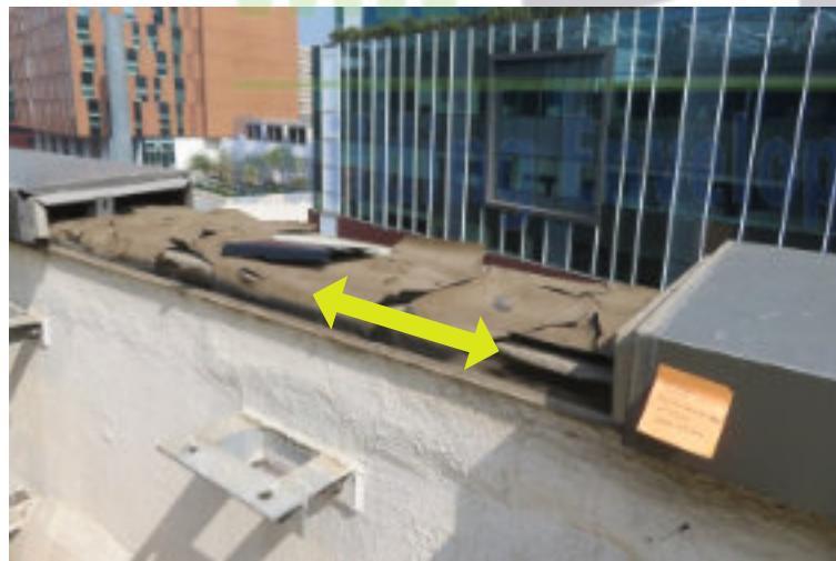
Waterproofing layer weathered out, lead to seepages
